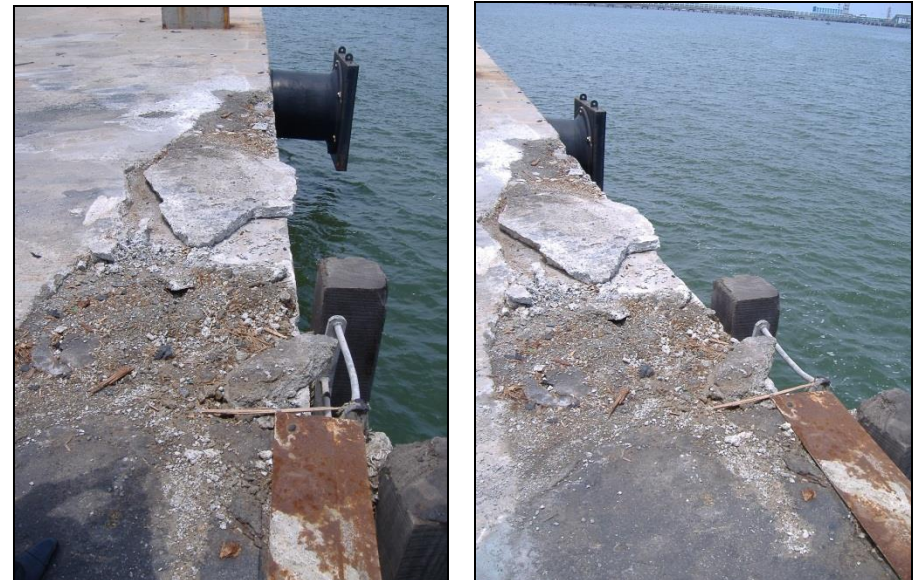
Damaged GCB by swell
