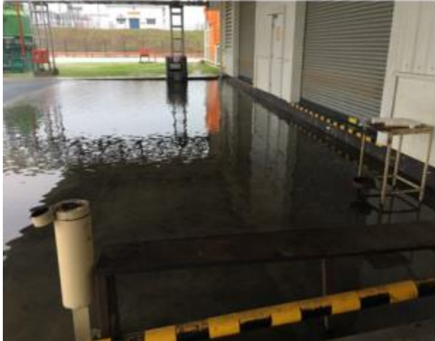
Water intrudes into building
